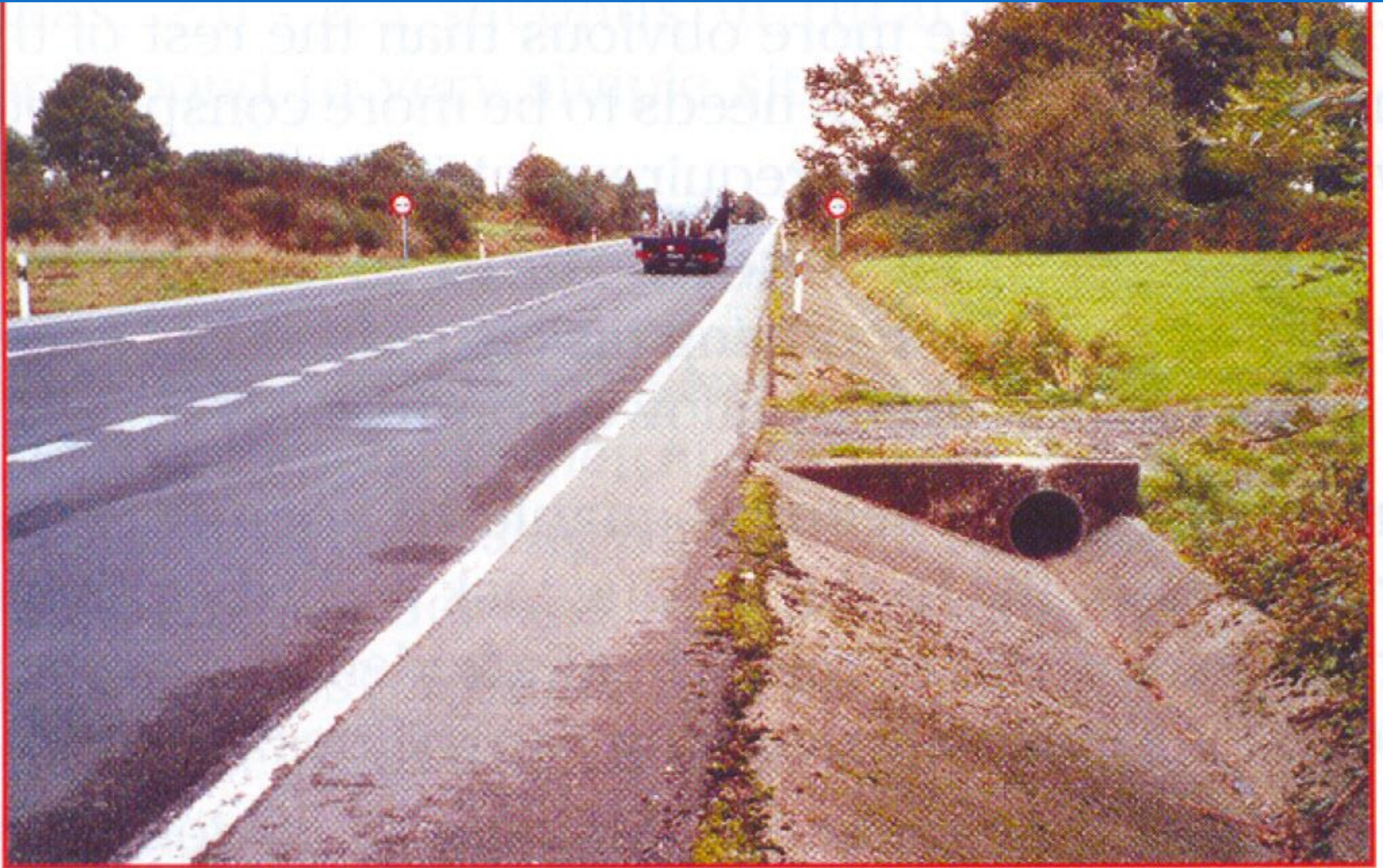
Hazardous drainage structure on a main rural highway (errant vehicle are directed on a vertical concrete structure)
